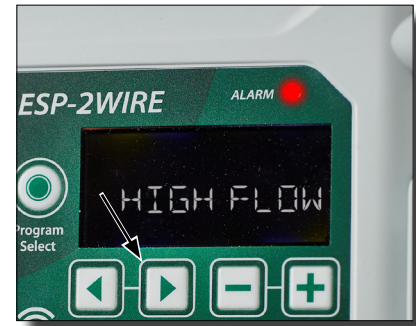
ESP-2WIRE Controller Front Panel High Flow Condition - Alarm
