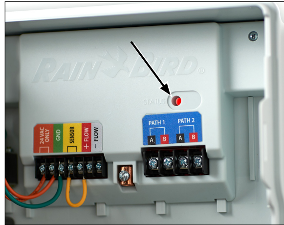
ESP-2WIRE Controller back plane
