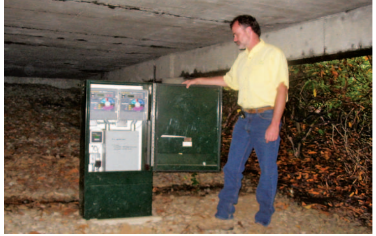
ABOVE: This enclosure holds two Rain Bird controllers that adjust watering rates based on data supplied by the Maxicom ET-data network. Project contractor Art Meisner shows off the unit, which is tucked under a patio where it is easily accessible.
