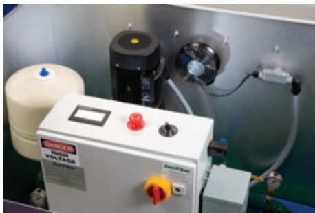
Interior of Low Profile Pump Station (LP)
