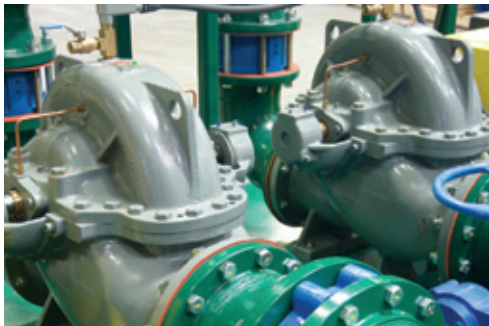
Water Feature Pump Station
