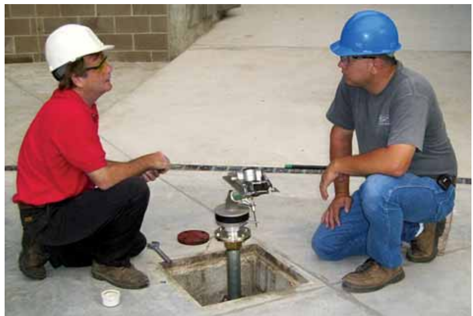
Mike Caldwell and John Kearns perform a routine system check to maintain optimum Rain Gun performance.
