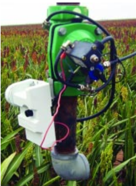
Close up of the Rain Bird Cast Iron Valve and Cyclik module.
