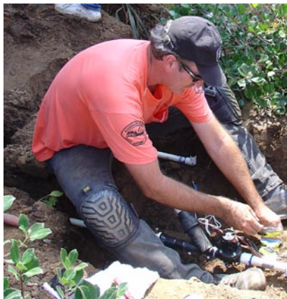
Dave Matthews installs Rain Bird's XCZ-100 Control Zone Kit. This medium-flow kit, with its durable DV Valve and RBY Filter provided an ideal solution for the new drip irrigation design.
