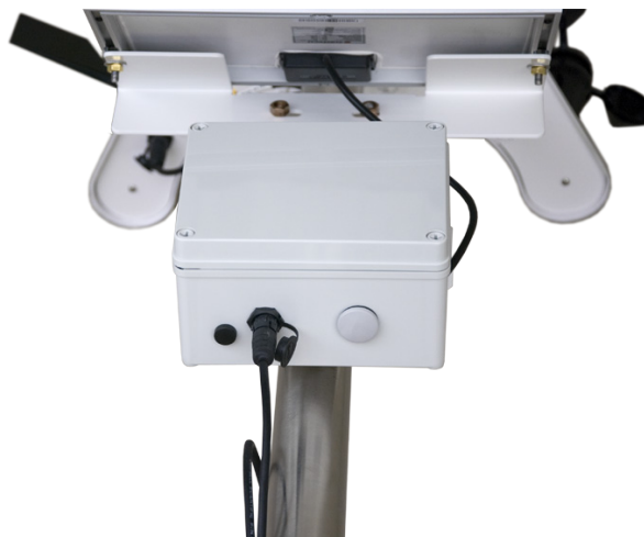
FIGURE 5-22. 18971 cable connected to auxiliary battery enclosure
