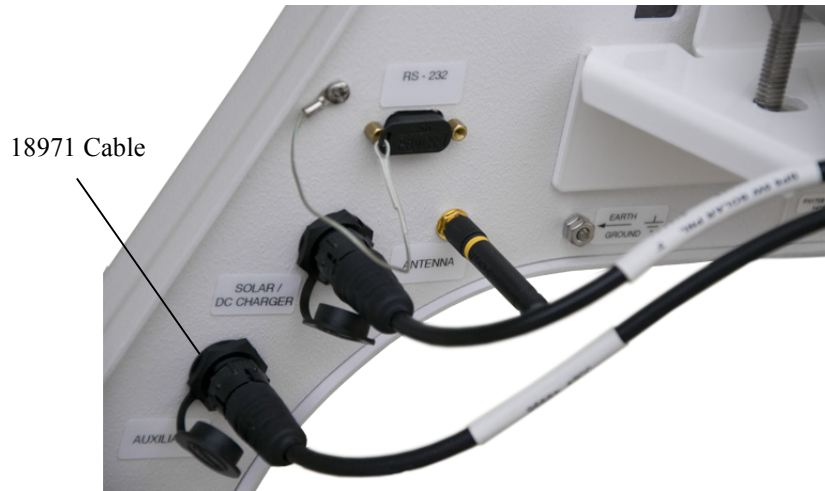
FIGURE 5-23. 18971 cable connected to WS-PRO LT station
