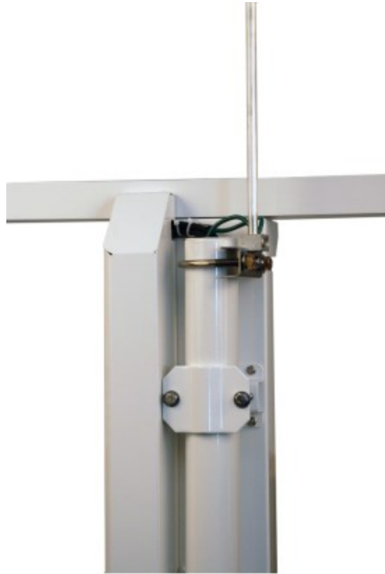
FIGURE 6-47. Connector cover in place
