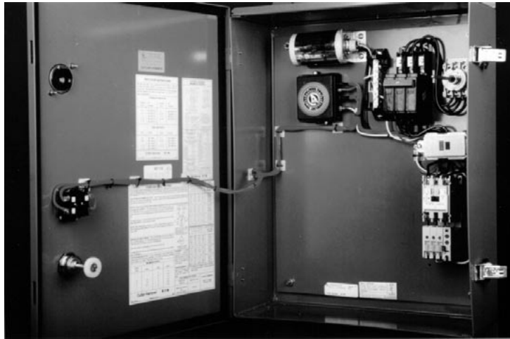
Power Control Center Open
