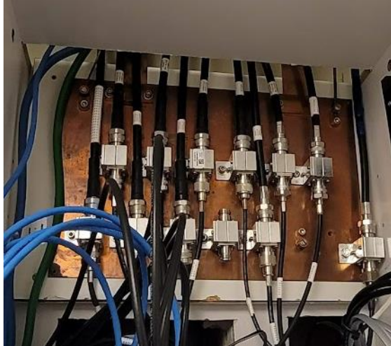
Example of multiple Polyphasers installed on OEM grounding plate
