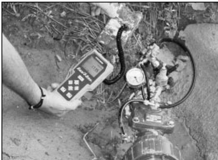
This control module and valve were buried for 2 weeks due to flooding. Infra-red communication with the field transmitter still worked.
