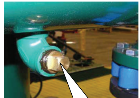
Figure 4 Example Pump Station Drain Plug
